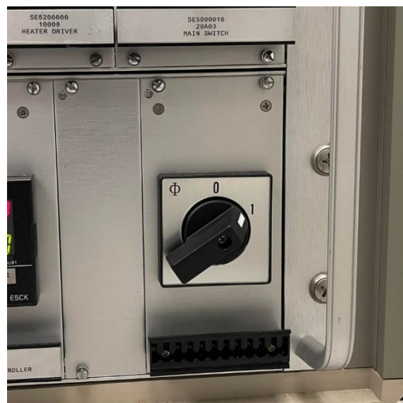
Figure 2. Heater Power Switch for EVG 501
