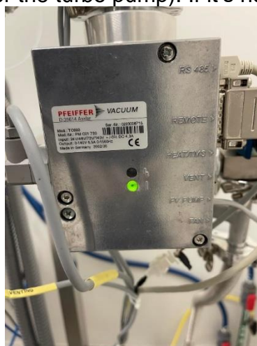
Figure 27. Turbo pump power supply in working condition.
