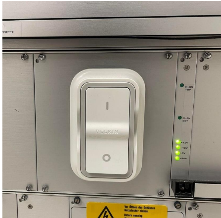
Figure 3. Roughing Pump Power Switch for EVG 501
