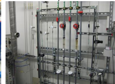
Process systems rack
